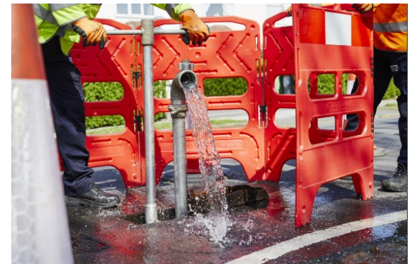
Pro-active leak detection
