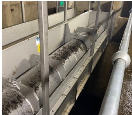
Combined Sewer Overflow in Rivadale
