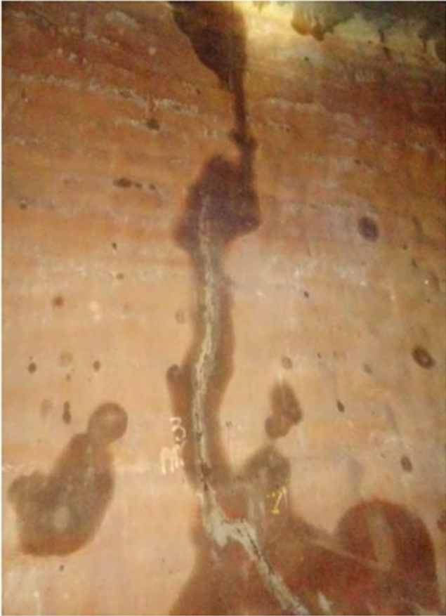
Figure 7.7 An example of the vertical cracking evident to the walls of Chellow E CWT
