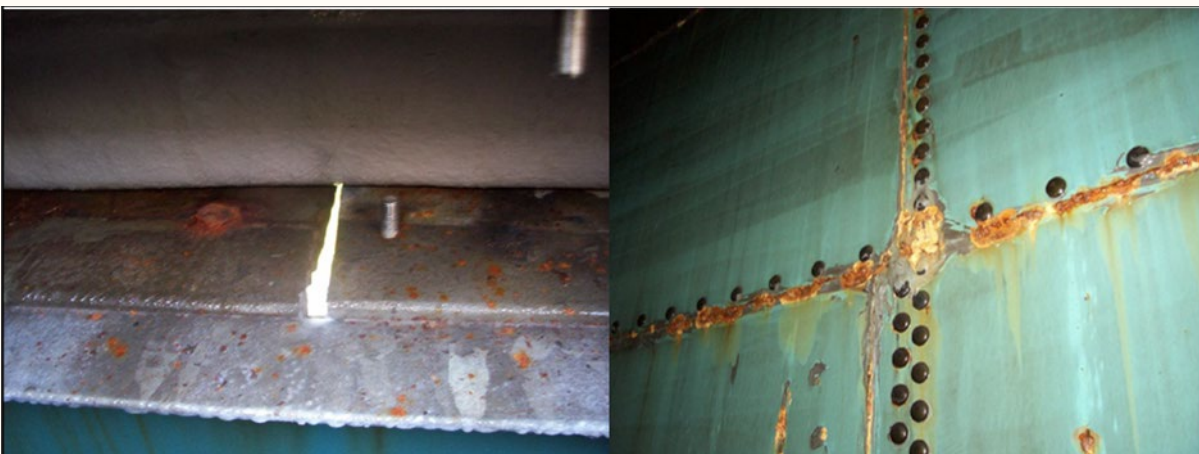
Figure 7.9 Thornton Moor integrity failures (routine inspection, 2009)
