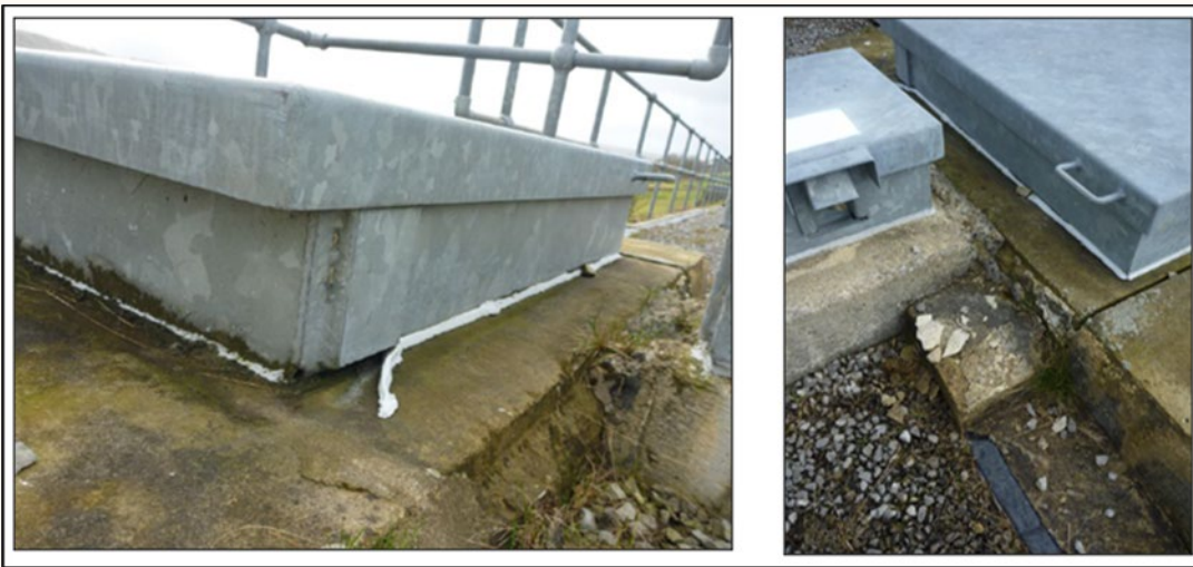
Figure 7.10 Bracken Bank ingress pathways and overall poor condition
