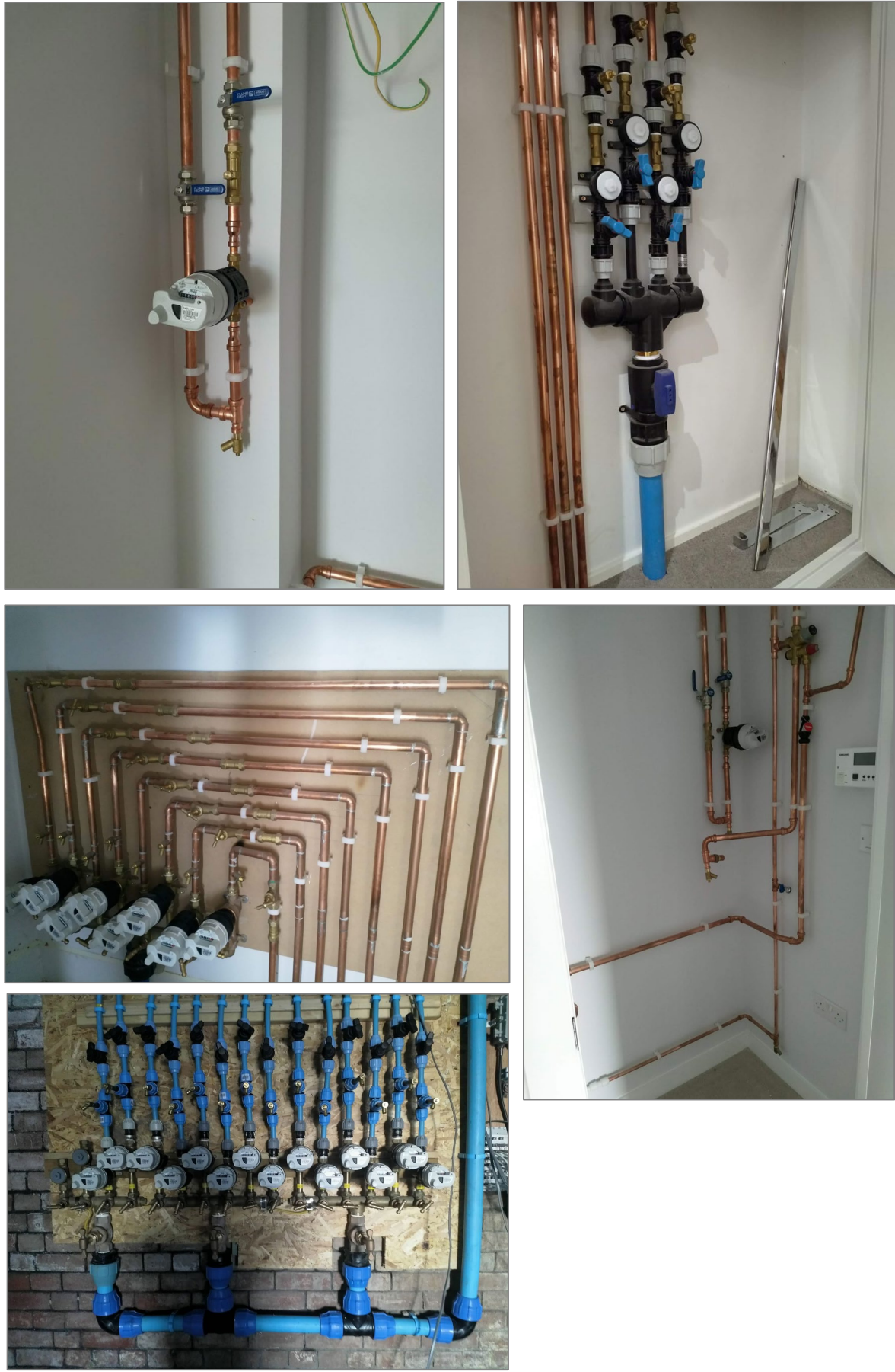
Figure 12: Internal Meter Fit Photos
